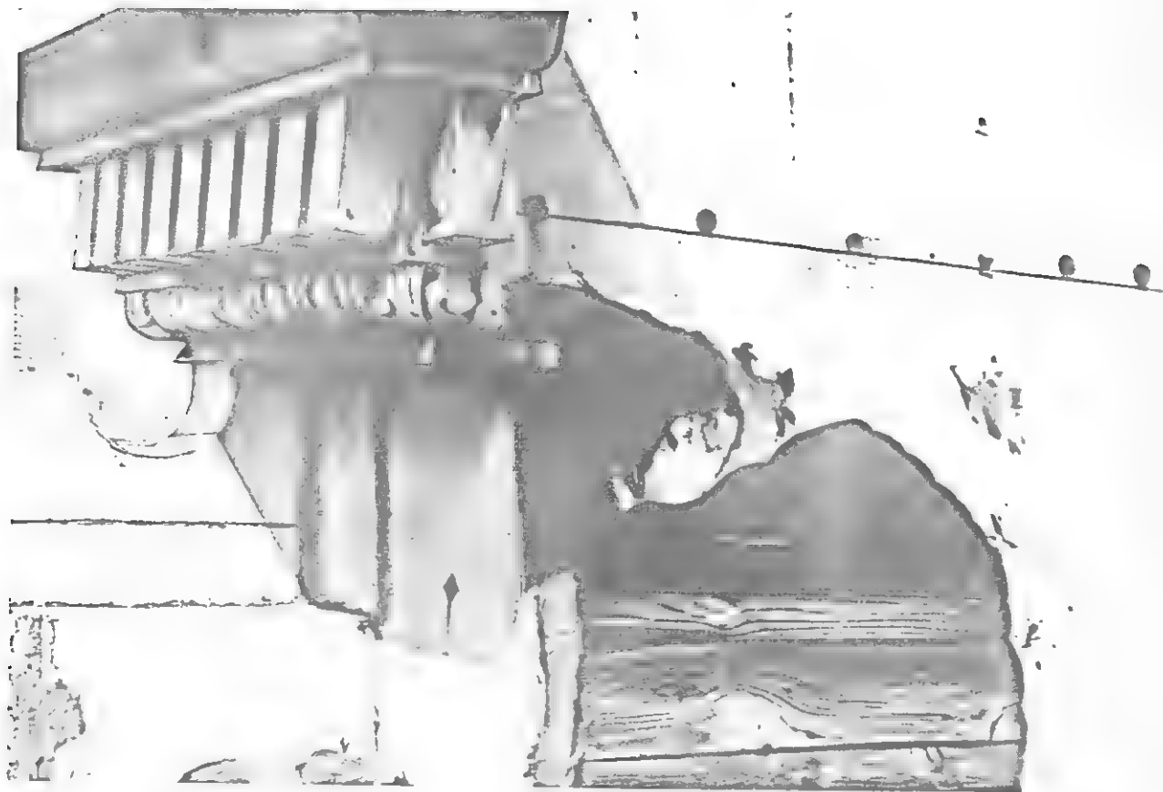
Back of segmental arch of parapet of northern facade of waiting room. This detail shows evidence that copper sheathing has been cut away.
